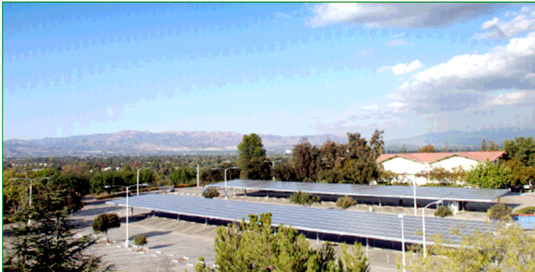
Pierce College, Woodland Hills – 191 kW dc solar power system
